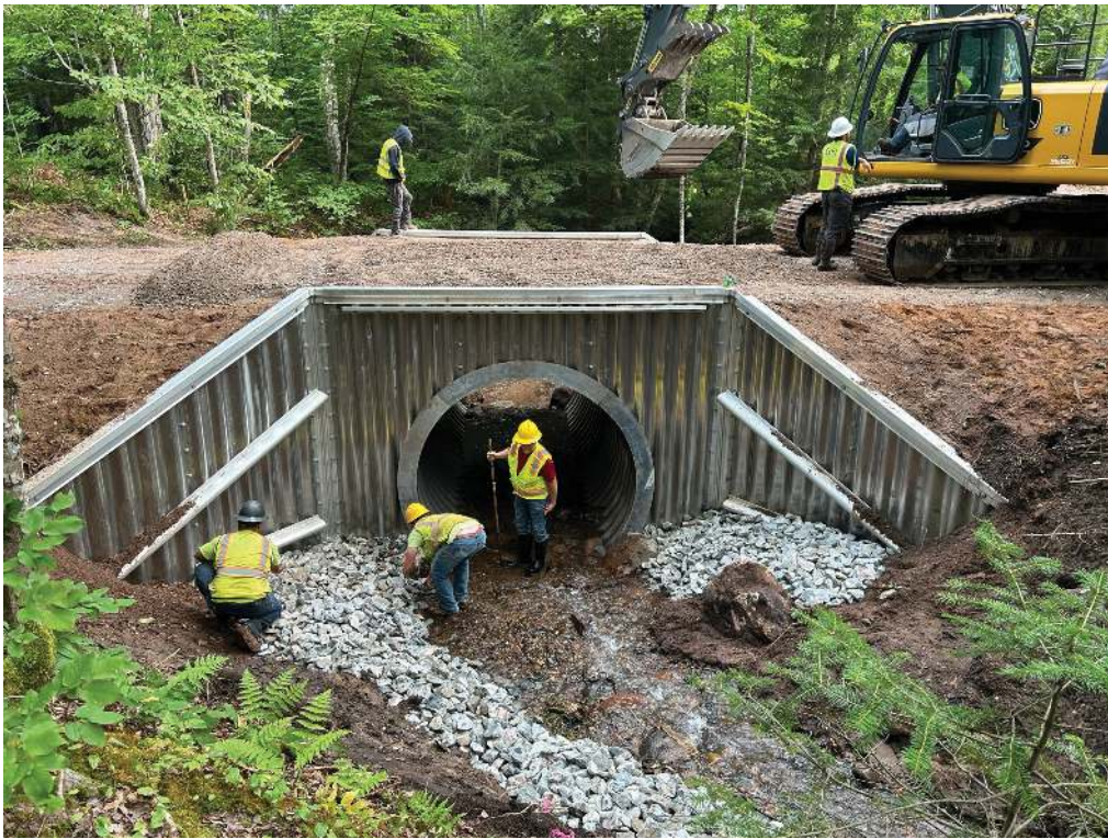
Mitch Koetje (center of culvert), working alongside the Ultra Construction crew during the final stages of installation. Photo by Sam Prentice.
