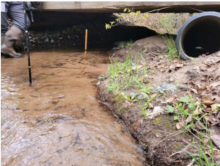
Before restoration: Creek bed is full of sediment and the old culvert is non-functional. Photo by Mitch Koetje.
