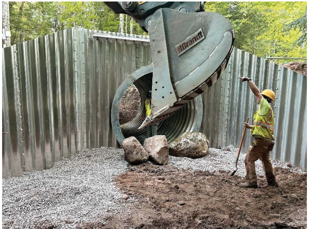
Ultra Construction installing the new culvert at the Deer Creek crossing. Photo by Sam Prentice.
