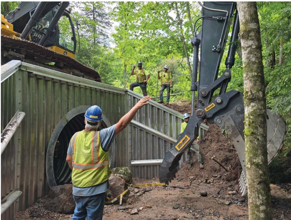
Bill LaForge of Ultra Construction guiding machine operator Todd Taskila during construction. Photo by Mitch Koetje.
