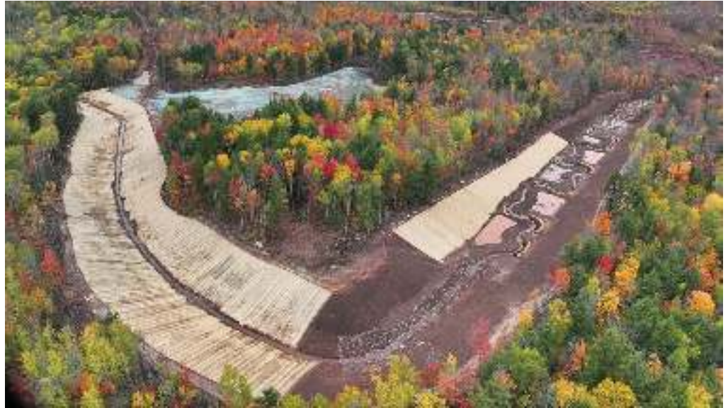
Stream diversion around future site infrastructure at Copperwood. Photo by Highland Copper.
